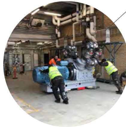
Gothenburg heat pumps
